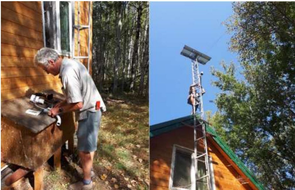
Left: Pete Kershaw setting up the new weather station. Right: Pete risks life and limb to install the station!
