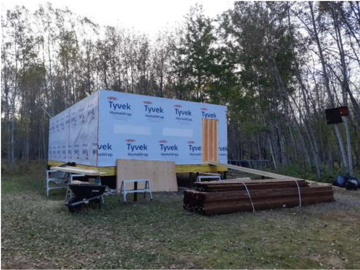
Construction is well underway! The first floor is built and construction crews will start on the front deck and second story shortly.
